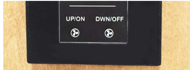
Power Roof Ventilator Switches
