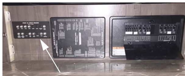
House Circuit Breakers -Typical View
