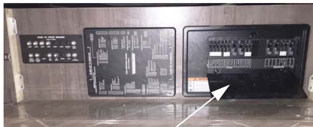
House Circuit Breakers -Typical Installation
