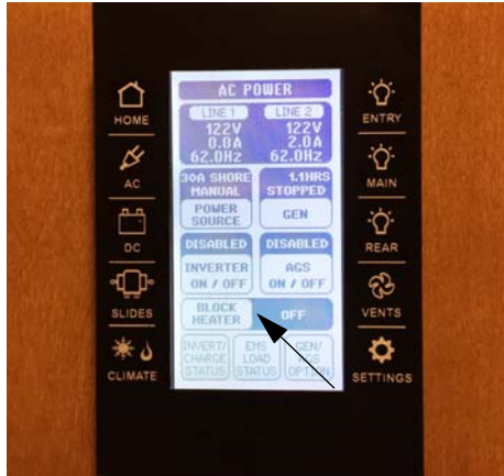
Diesel Engine Heater Switch (Located on multiplex monitor panel)
