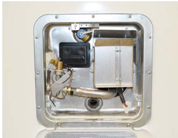
Water Heater Exterior Service Access
