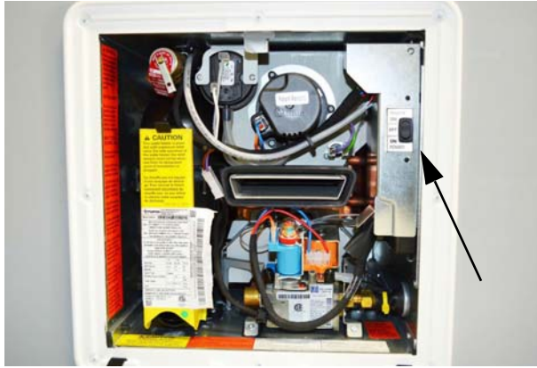
Water Heater Power Switch (Located behind water heater access panel on exterior of the motorhome)
