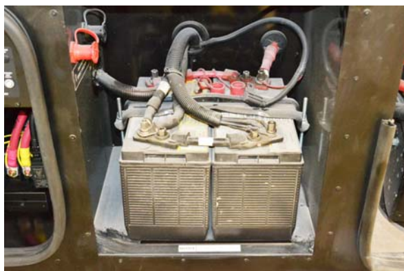
Chassis Batteries -Typical View
