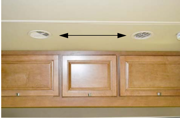
Supply/Return Air Vents (Located throughout the ceiling of the motorhome) -Typical View
