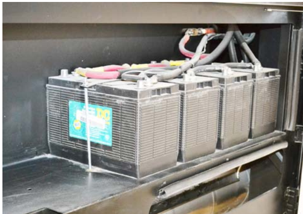
House/Coach Batteries -Typical View
